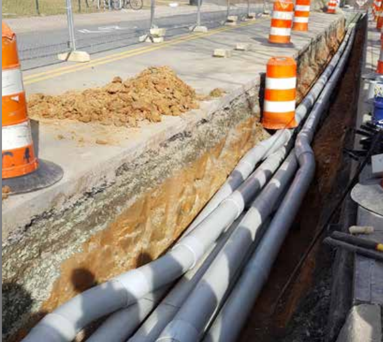
With most of the ductbank route set along active roadways, maintenance of traffic and pedestrian detours were critical to minimize impact on motorists. Photo: Dewberry
