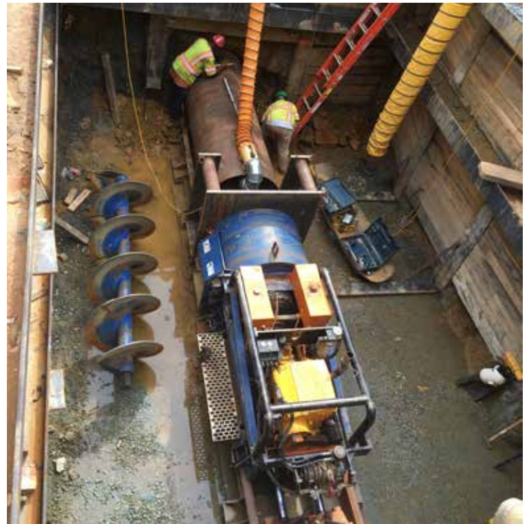
A jack-and-bore process allowed for ductbank installation along a busy street without closing the street to traffic. Photo: Dewberry
