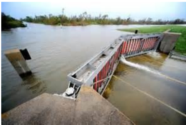
Figure G-14 - Gate Controlled Diversion Structure
